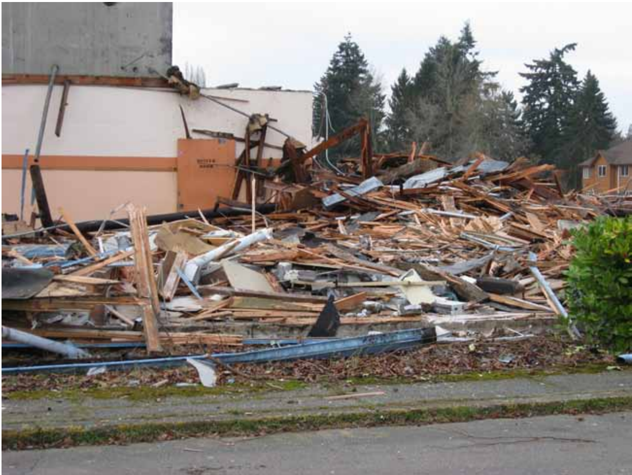
Figure H-6. Partially Demolished Building to be Loaded in an Intermodal Container
