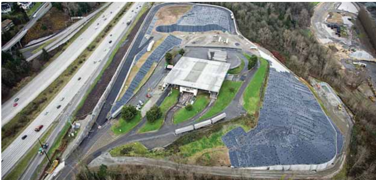
Site work has been completed for the new Bow Lake Recycling and Transfer Station.
