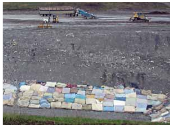
Mattresses act as a filter to keep sediment out of the drain layer material in the new Area 7.
