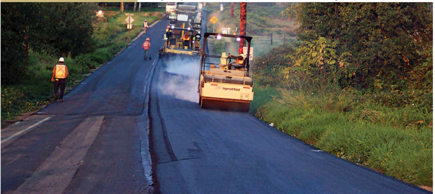
A King County road near Enumclaw is paved in 2009 with HMA containing RAS and RAP.
