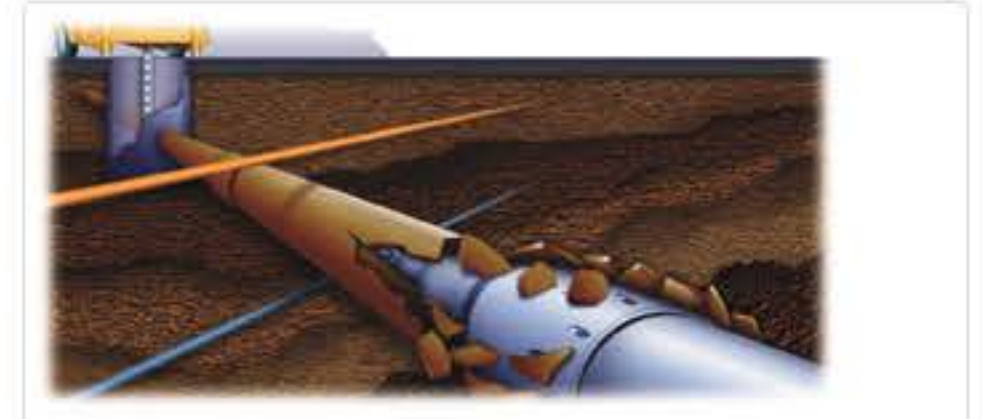
A pipe cutter breaks up an existing pipe while pulling another pipe behind the expander head.
