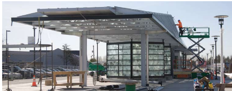
A construction worker at the Burien Transit Center in March, as the center neared completion.
