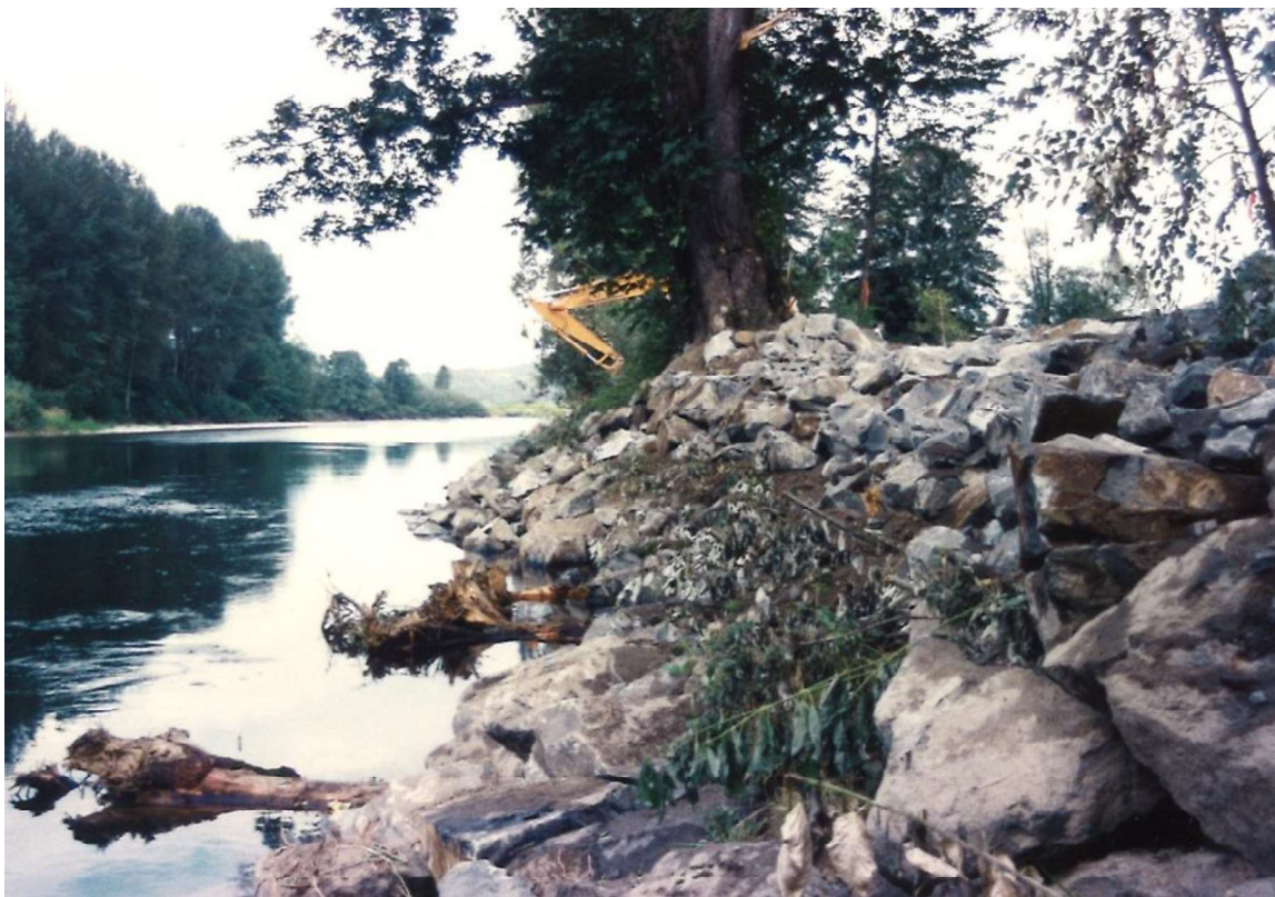
Figure 11 – Photograph of the 1997 repair of the Haffner Revetment, which included bank embedded wood near the summer low flow water elevation.
