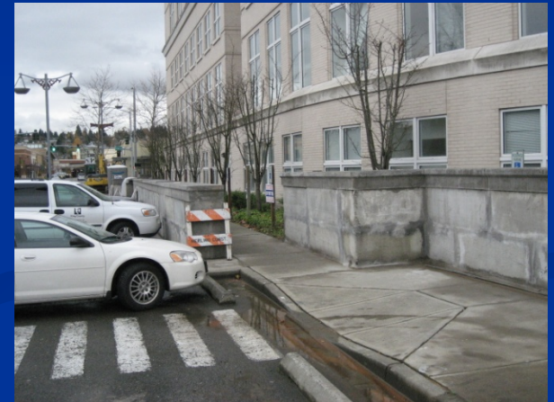
Ecology Block Wall – MRJC
