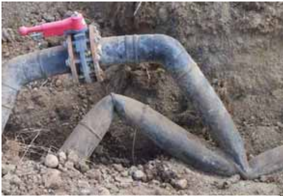
LFG Pipe Buckling Failure
