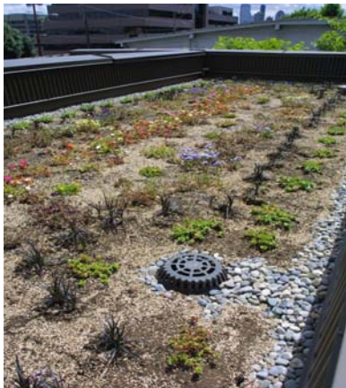
The Dexter-Horton Regulator Station's Green Roof
