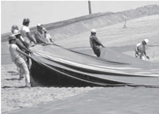
▲ Liners installed during the construction of new disposal areas preserve the quality of our environment
