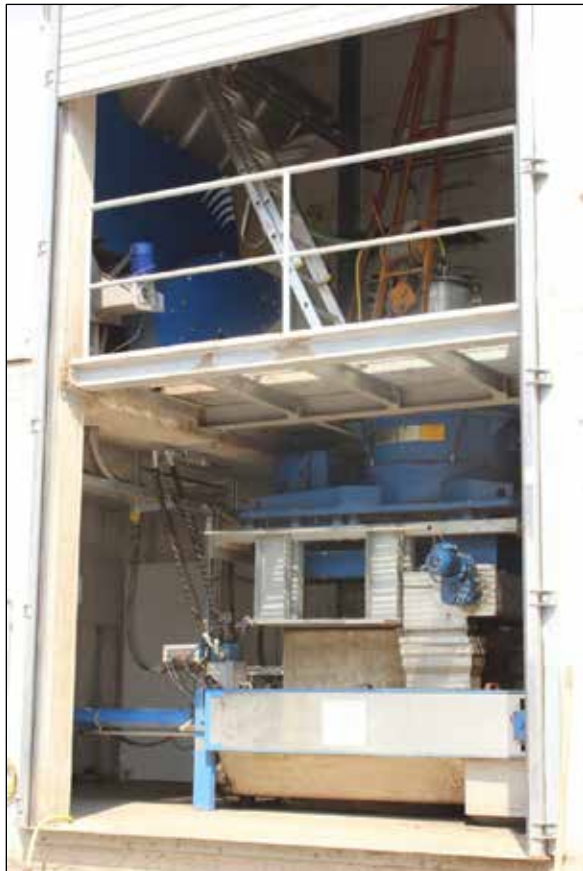
Figure 3-5. FITEC, Rothmuhle Biogas Plant: Biosqueeze Unit
