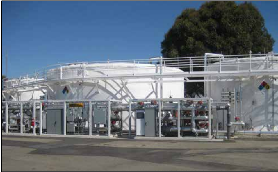
Figure 3-15. Clean World Anaerobic Digestion Facility in Sacramento, California
