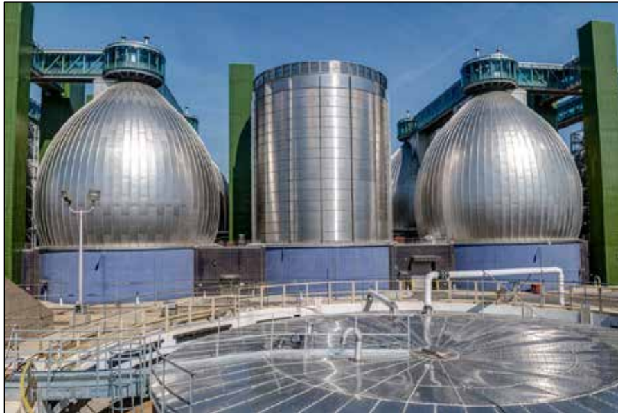
Figure 3-11. The NYCDEP WWTP Anaerobic Digesters
