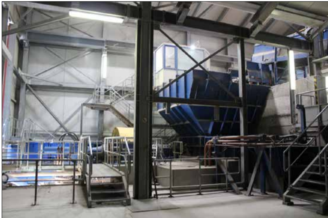
Figure 3-7. Anaergia, OREX, Kaiserslautern: Feed Hopper (right), OREX Press (bottom left)
