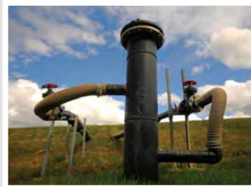
The landfill gas management system includes extraction wells that prevent gas from leaving the site and probes that detect the movement of gas. The system is designed to prevent landfill gas from escaping from the site.
