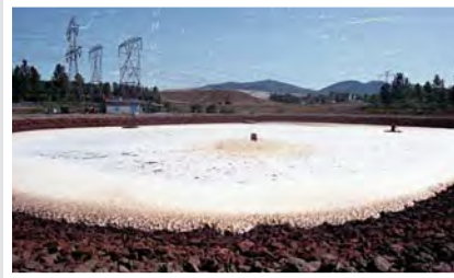
In the late 1970s, a leachate collection system is constructed. Leachate – produced when water percolates through garbage – is collected in pipes and diverted to on-site aeration ponds, where it is pretreated before being sent to a wastewater treatment plant.
