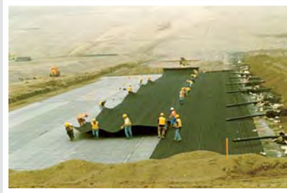
The bottom liner and clay barrier prevent leachate from seeping into the soil or groundwater.
