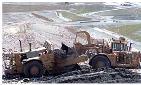
In 1986, the landfill achieves full daily cover, meaning six inches of compacted soil is used to cover the entire surface of the active solid waste disposal area at the end of each working day. Daily cover serves to control litter and discourage foraging by animals.
