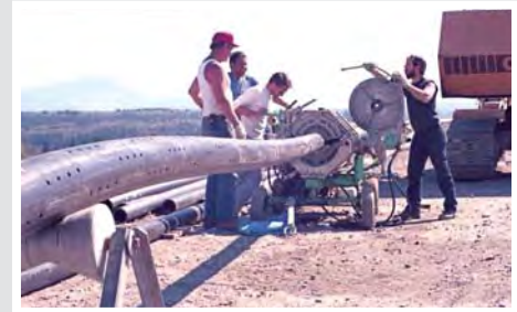
The leachate collection system has been continuously expanded since its birth in the late 1970s.
