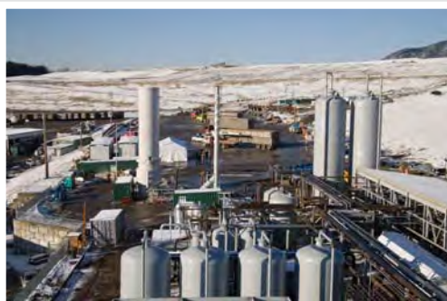
In 2009, a landfill gas-to-energy facility begins operations to convert the landfill gas into pipeline-quality natural gas. The renewable energy produced by the plant each year equals the amount of energy needed to meet the natural gas needs of over 19,000 homes in King County.
