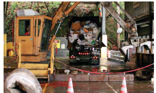
Commercial and self-haul customers dump directly into the refuse trailers located in the trailer tunnel, under the chutes, from the tipping floor above. A stationary compactor is used to distribute and tamp the material in the trailer.
