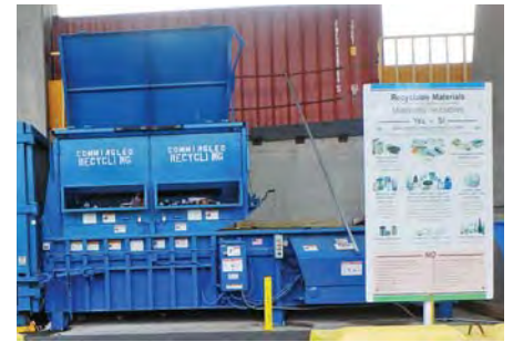
Compactors for recyclable materials
