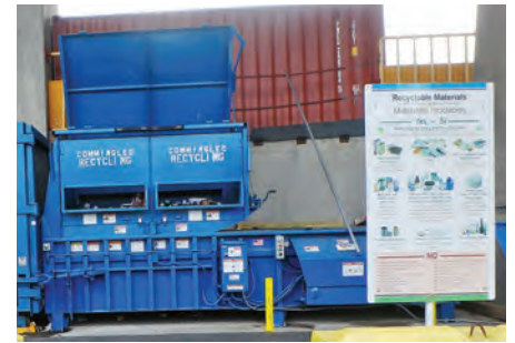
Compactors for recyclable materials
