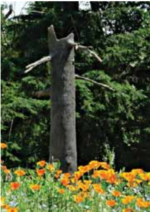
Hidden Lake Pump Station Replacement – Odor Control Stack Disguised as a Tree Snag
