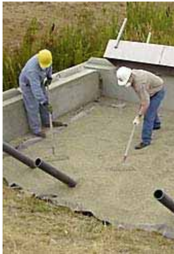
King County employees install VitroClean crushed glass filtration media in the stormwater filter vault at the Auburn Park & Ride.
