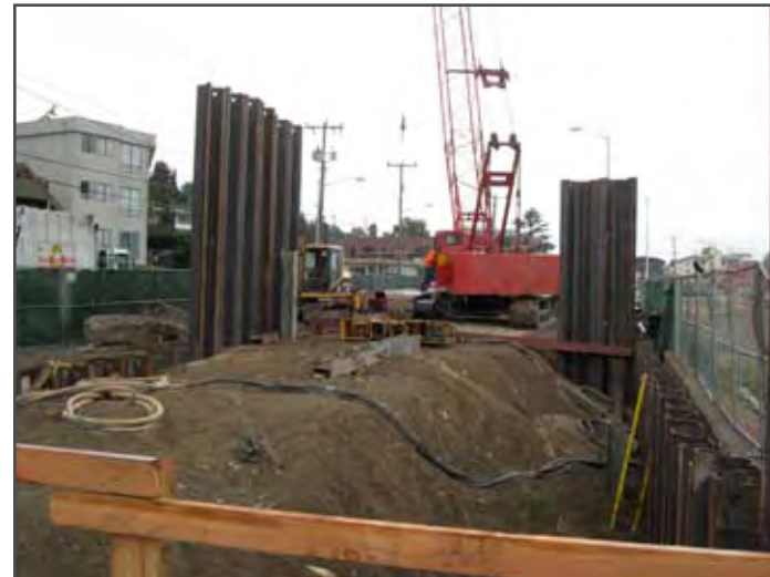
The crane and a vibratory hammer vibrating sheet piles into the ground.
