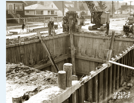
Construction shown here in 1953 at the site of the original pump station looks similar to construction today as we expand the pump station. View more photos inside.
