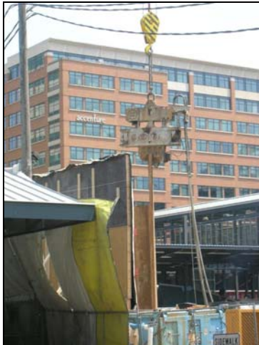
Vibratory hammer and sheet pile suspended from crane at the King Street Odor Control Project.
