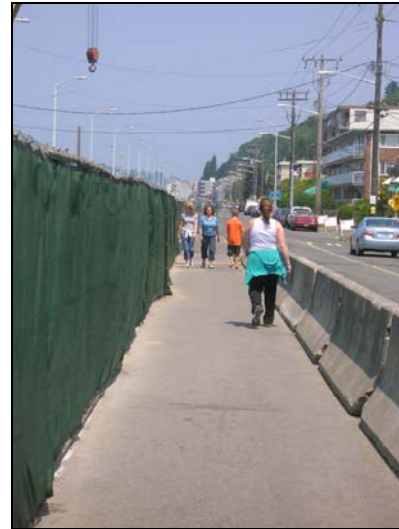
Pedestrians on the new path between the construction zone and Alki Avenue Southwest.
