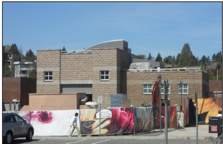
Exterior improvements are nearing completion on the Kirkland Pump Station located at the corner of Park Lane and Third Street.
