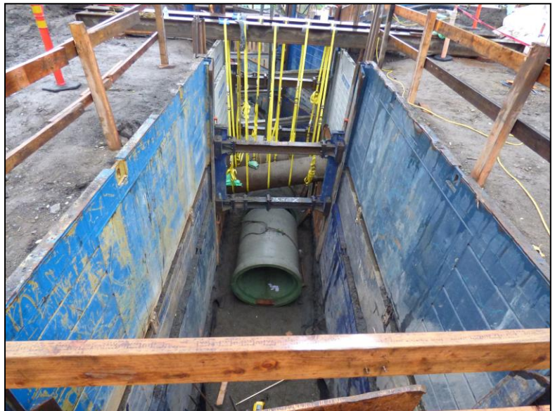
Installation of the final section of the 5-foot-wide sewer pipe will begin as early as May 12.
