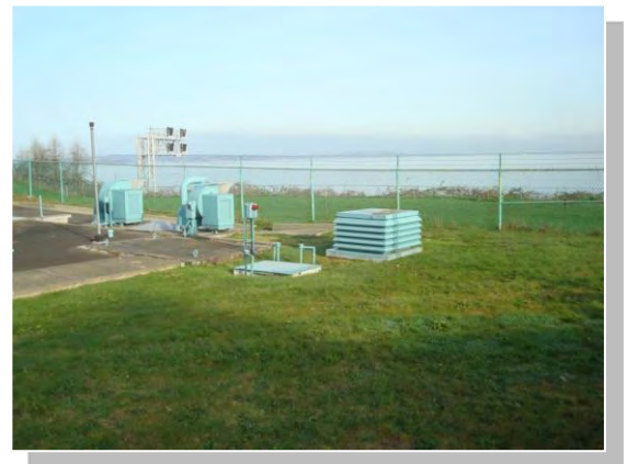
King County's North Beach Pump Station
