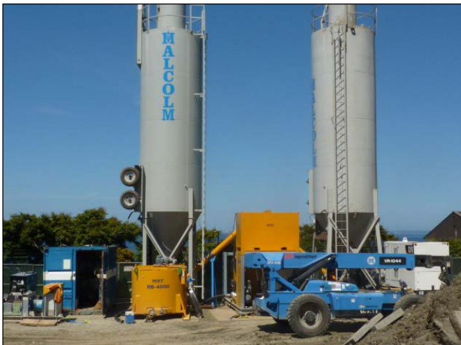
Specialized grout is made on-site in the batch plant. Grout is made on-site to ensure a grout mix of the quality and specification required.
