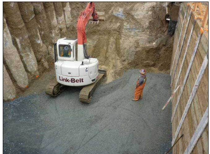
Excavation for the new mechanical/electrical building has begun. After the area is excavated, a concrete foundation will be poured.
