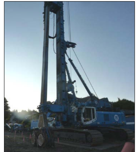
The drill rig (CSM machine) used to create panels for the shoring system for the combined sewer overflow (CSO) storage tank. Read more on the back.
