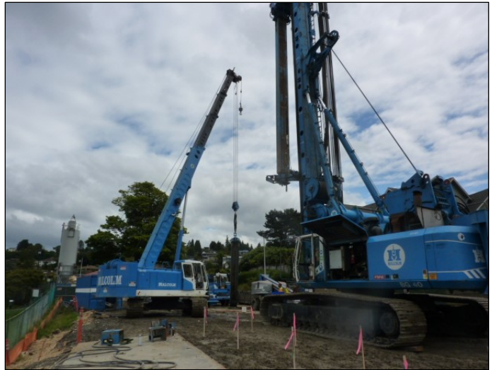
The crane inserts a beam into the shoring panel, before the grout mix cures and hardens. Each panel must be completed once it has been started.
