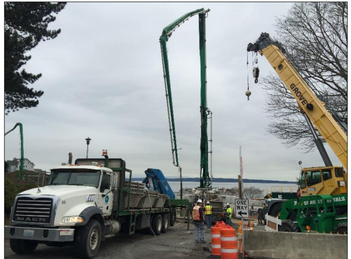
The contractor poured 300 cubic yards of concrete on Monday, continuing to form the CSO tank base.
