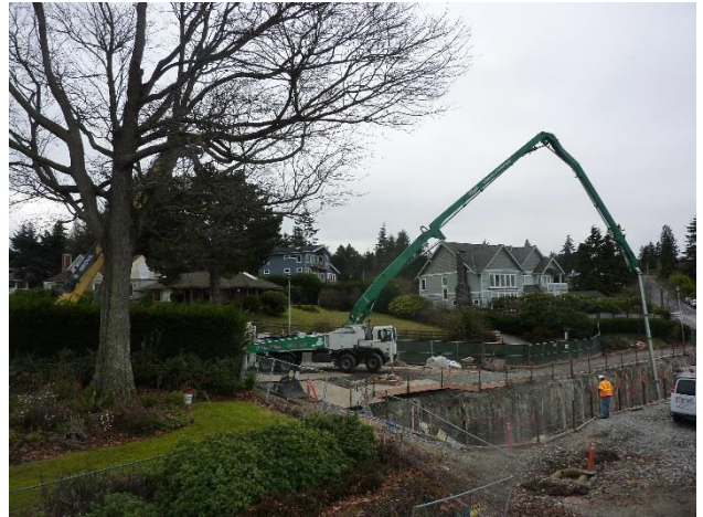
The contractor completed pouring concrete for the base of the CSO tank on Tuesday, December 23.
