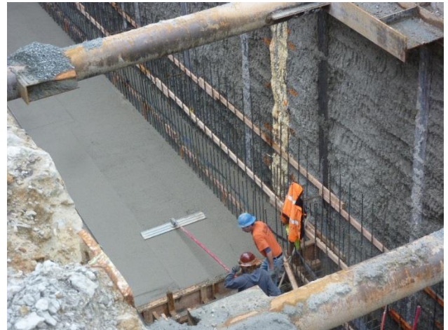
Crews finish a section of the CSO tank slab after the concrete is poured.
