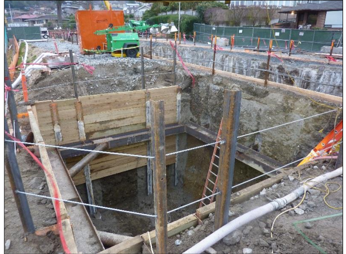
Construction of the 48b structure continues. The 48b structure serves as a backup for CSO discharges when the North Beach Pump Station can't get all flows to Carkeek Park or through the main outfall.
