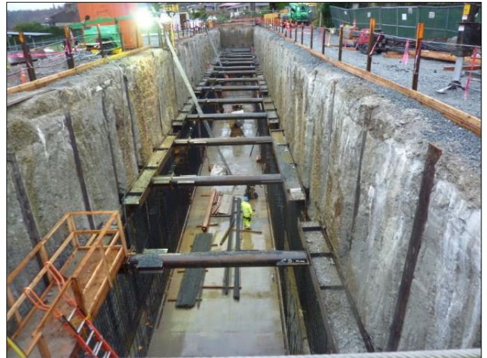
Progress continues on the CSO storage tank. This photo is from January 5.
