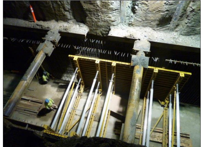
Progress continues on the CSO storage tank. This photo is from January 13. Crews are installing the tank wall forms, in preparation for concrete pours.
