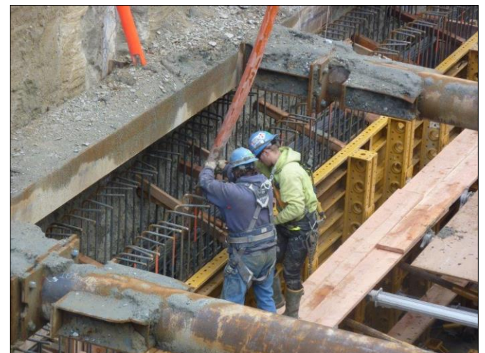
Crews pour concrete through a pump to form a wall of the tank.
