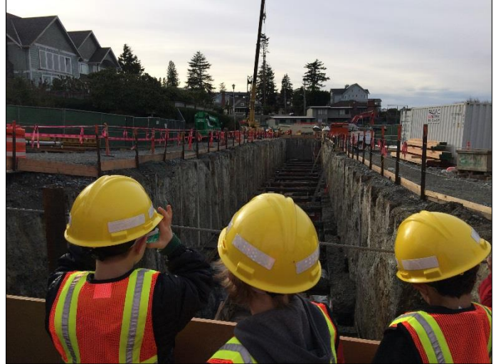
Second graders from North Beach Elementary look into the tank excavation area during a site tour on Wednesday.
