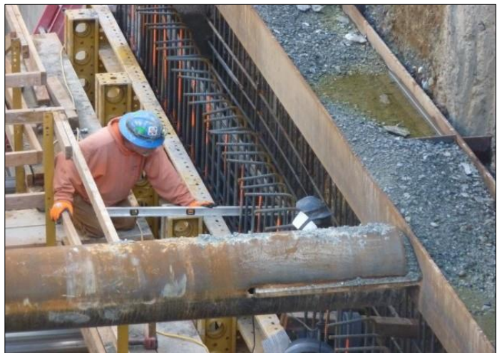
Crews install forms, which are like molds, for the CSO tank walls.
