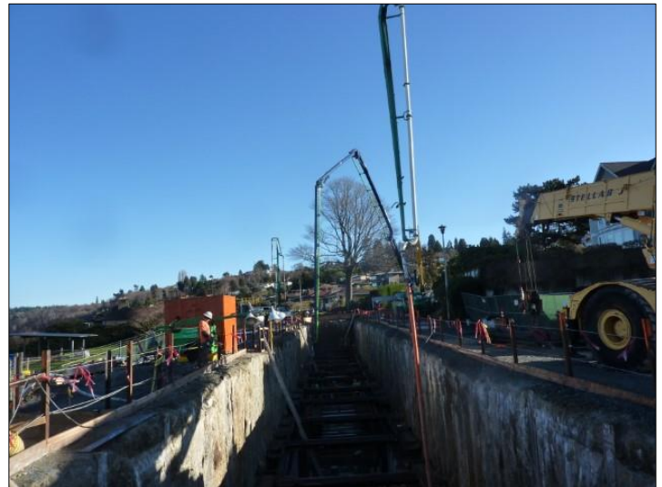
Concrete pourers reach deep into the CSO tank area to pour concrete for the tank walls.
