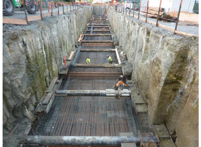
Crews place rebar for the top of the CSO tank in preparation for pouring concrete.
