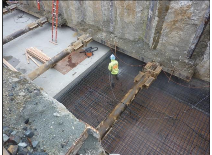
Crews forming the top of the CSO tank in preparation for pouring concrete.
