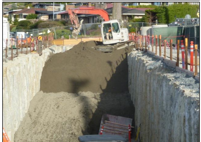
Gravel and soil (“backfill”) being brought on site to fill the CSO tank excavation.
