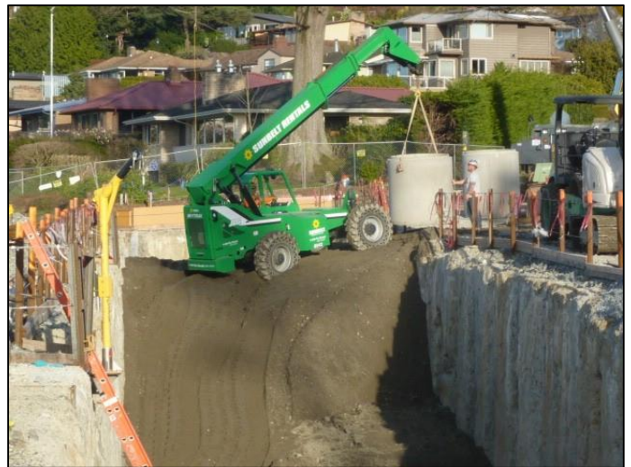
Crews continue to backfill the area above the CSO tank and will soon begin installing utilities.
