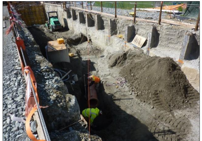
Crews install utility lines above the CSO tank, while continuing to backfill the tank area.
