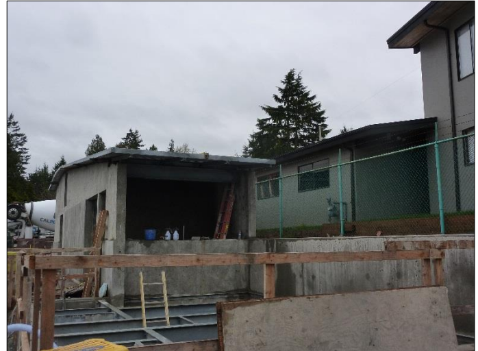
Work on the mechanical/electrical building continues, with the new roof almost complete.
