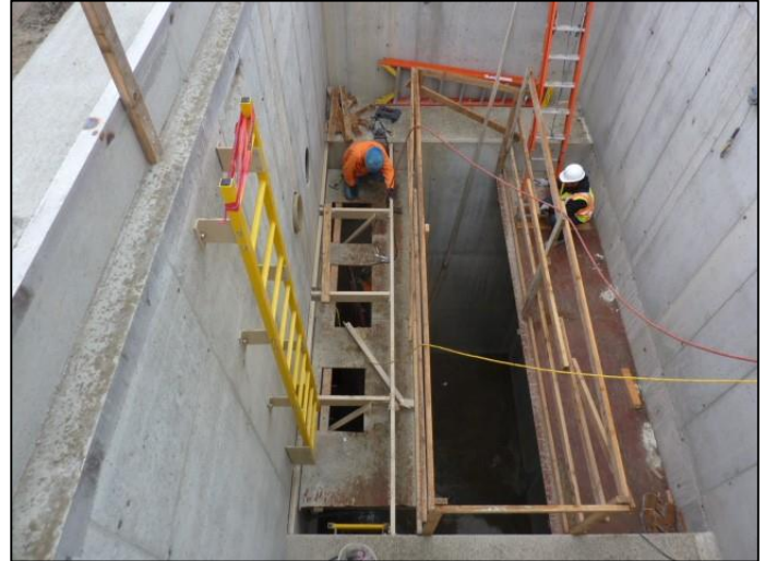
Crews work on the CSO tank “flushing vault” and tipping bucket, which will remove excess debris from the tank after a CSO event.
