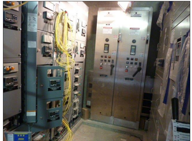
Electrical equipment inside the mechanical/electrical building.
