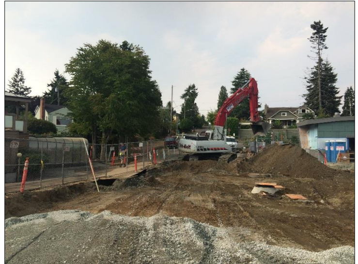
The construction site on August 12. The contractor digs to prepare for final paving.
