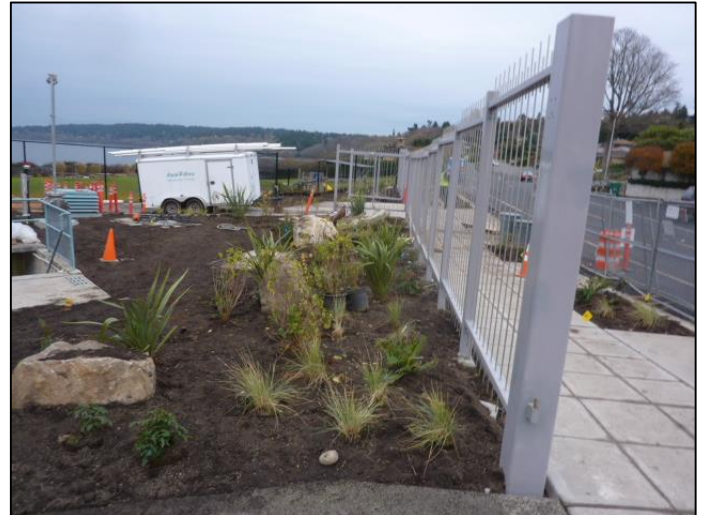
Landscaping and the new ornamental fence on the County pump station site.
