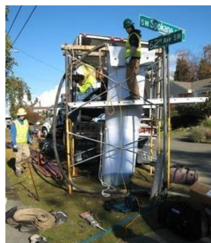
Sewer pipe liner being inserted at a manhole on the county's Beach Drive lining project in West Seattle.
