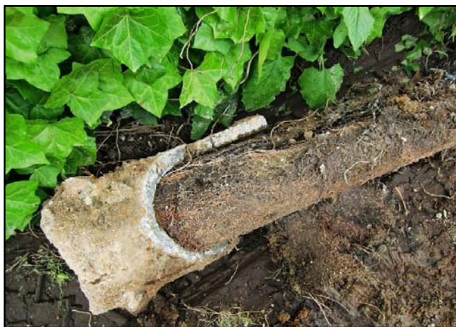
A side sewer blocked by tree roots
