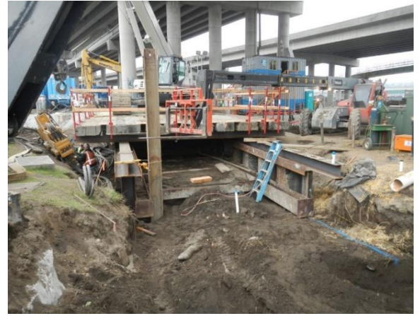
The trestle (shown above) will continue to be installed, eventually moving into the Duwamish River. It will be used to hold the crane and excavator needed for pipe installation.
