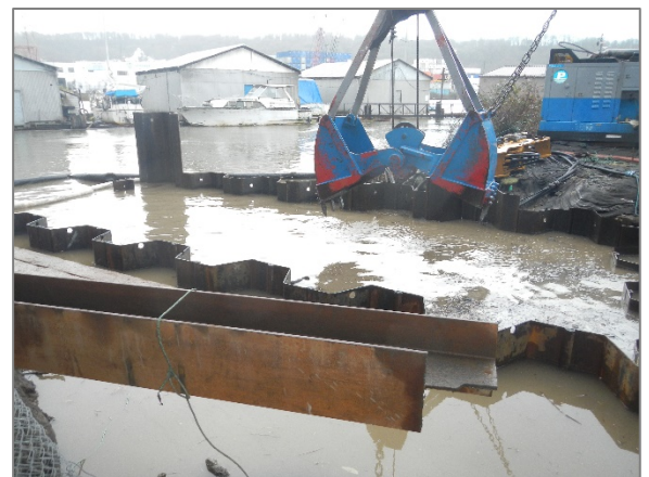
The contractor uses an excavator to prepare the riverbed at the outfall site.
