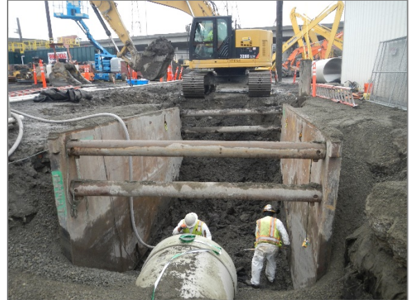
Crews use trench boxes to secure the excavation area while pipe is installed.
