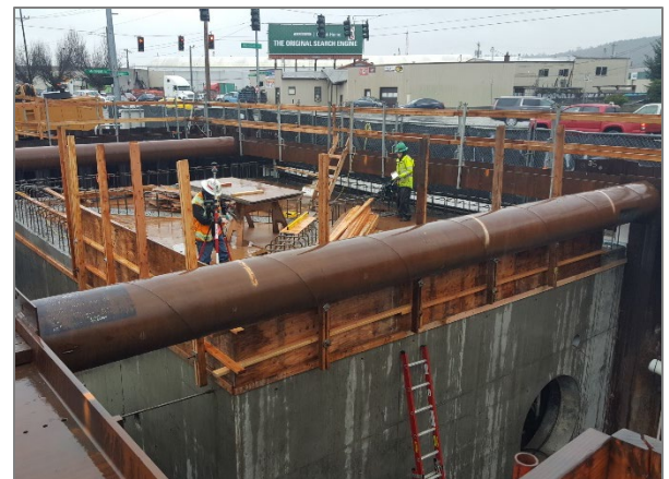
Crews working on the regulator structure, which will divert flows as needed during heavy rain events.
