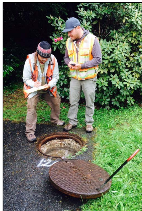
Crews working for King County survey the project area and check underground utilities.
