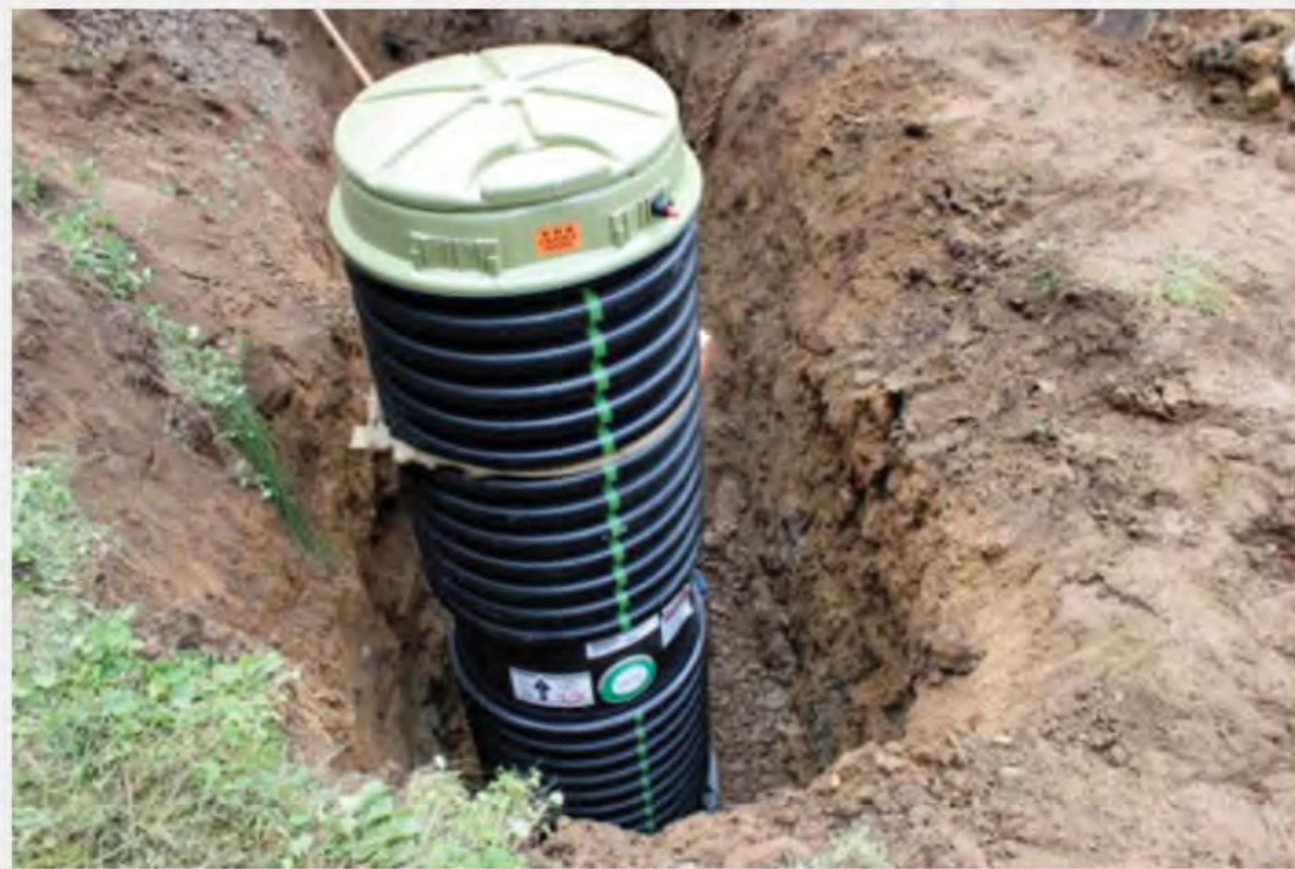
Example of a temporary bypass sewer system using grinder pumps
