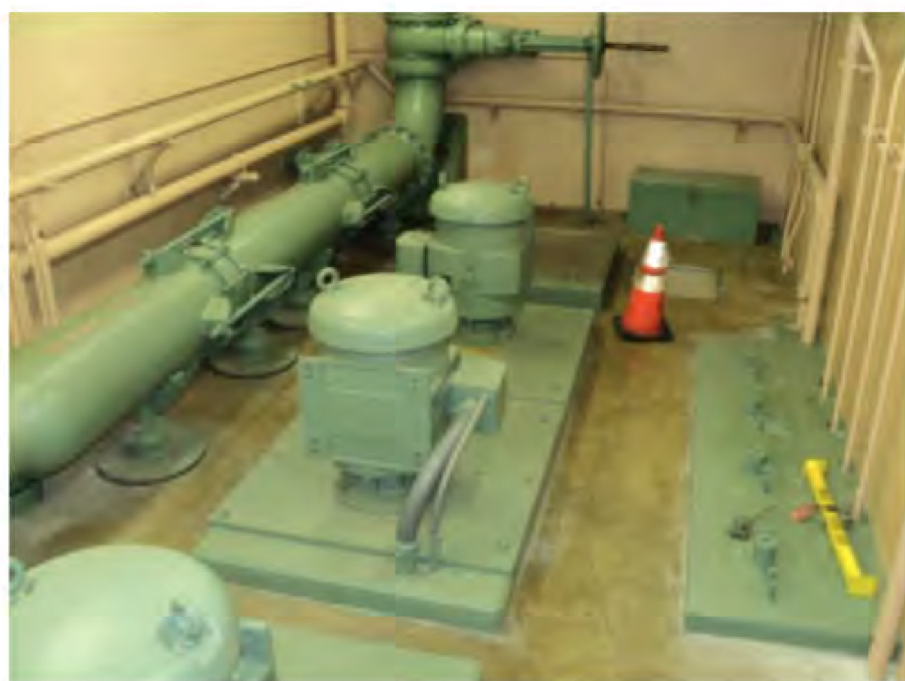
Interior of North Mercer Pump Station
