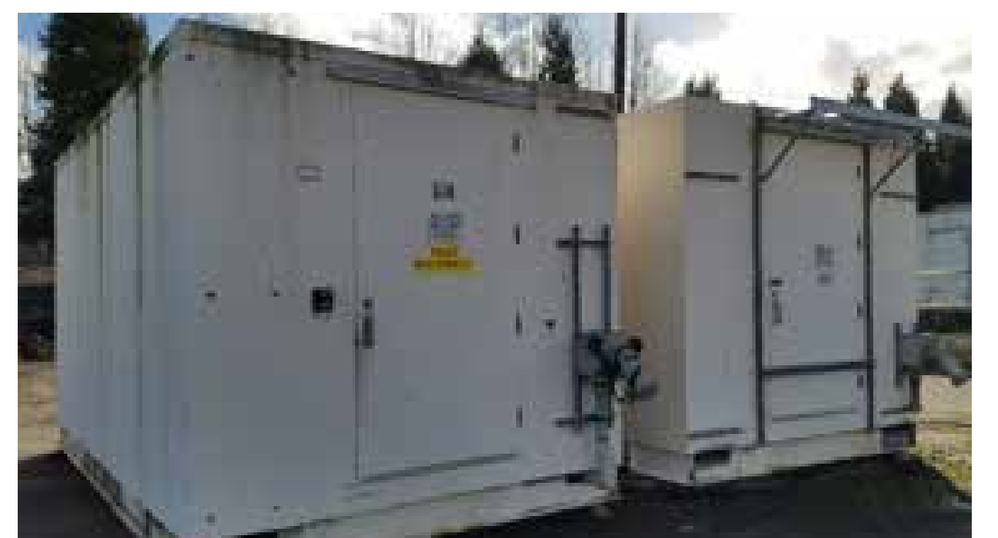
Power & Controls Trailers
