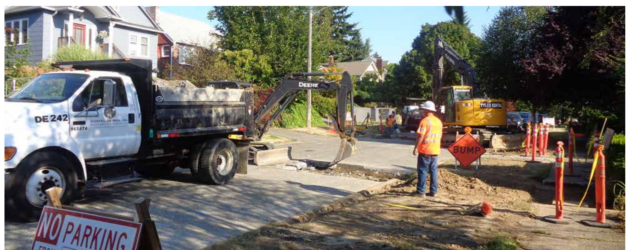
During construction, crews will place temporary ramps over the pipe to allow residents to access their driveways. Some mailboxes may need to be moved temporarily.
