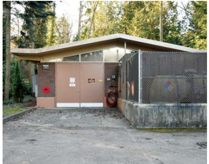
The existing North Mercer Island Pump Station (above)
