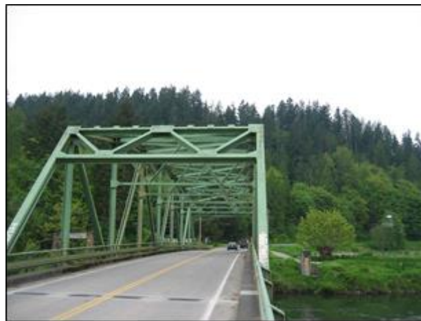
End portal of the Stossel Bridge over the Snoqualmie River near Carnation.
