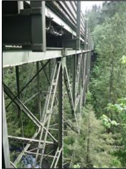
The Green River Gorge Bridge is King County DOT's only deck truss bridge.
