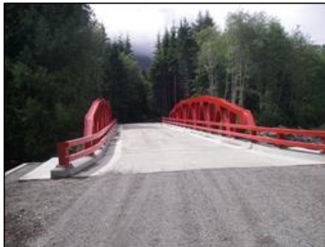
The Sunday Creek Bridge from 2010 is a pony truss bridge without height restrictions because of its open design.
