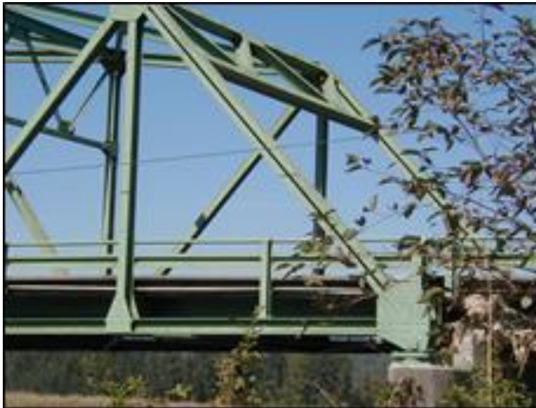
Signage will be placed at the portal to the through truss on the Stossel Bridge.
