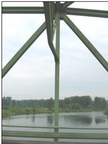
High load hits, such as this one on the Stossel Bridge, bend members out of plane. Heat straightening realigns the members to their original geometry without compromising strength.
