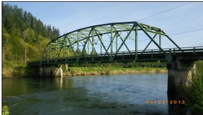
The Stossel Bridge has a through truss design similar to the span on the Skagit River Bridge.
