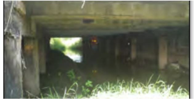
Mullen Slough is filling with sediment.
