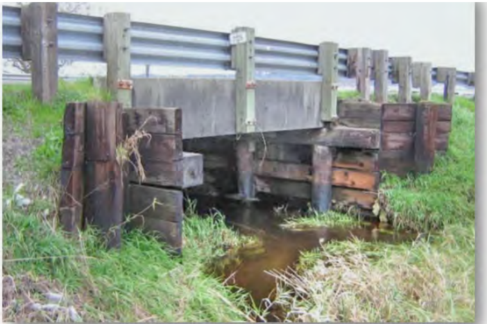
This bridge carries 24,000 vehicles each day, including 2,600 trucks and millions of tons of freight.
