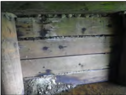
Sand is pushing through back walls.
