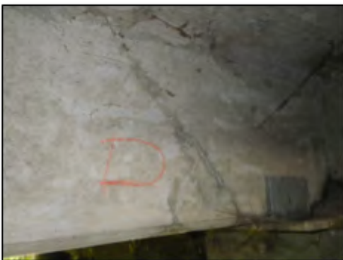
The concrete is cracking.
