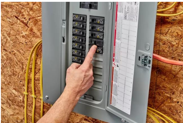
Figure 1 Electrical panel image. Source: How to Install a 240-Volt Circuit Breaker (thespruce.com)
