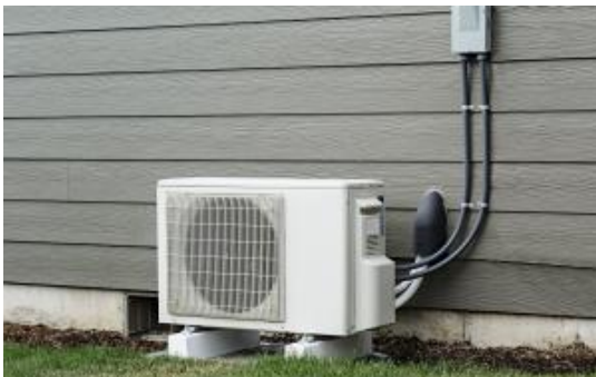
Figure 1 Ductless heat pump outside compressor. Image source: Ductless (Mini-Split) Heat Pumps | Building America Solution Center (pnnl.gov)
