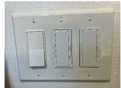
Figure 1 Dimmer capability for lighting on the middle and right switch (left switch controls a local exhaust fan).
